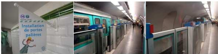
Figure: Synchronisation of platform screen doors - Paris Metro
