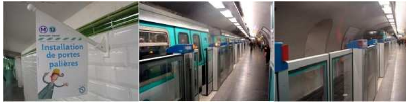
Figure : Synchronisation of platform screen doors - Paris Metro
